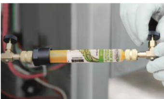
Charge inline with refrigerant
